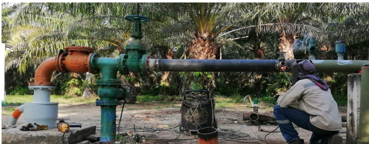
Figure 1-2. Ground water pump feeding the micro aspersion system
