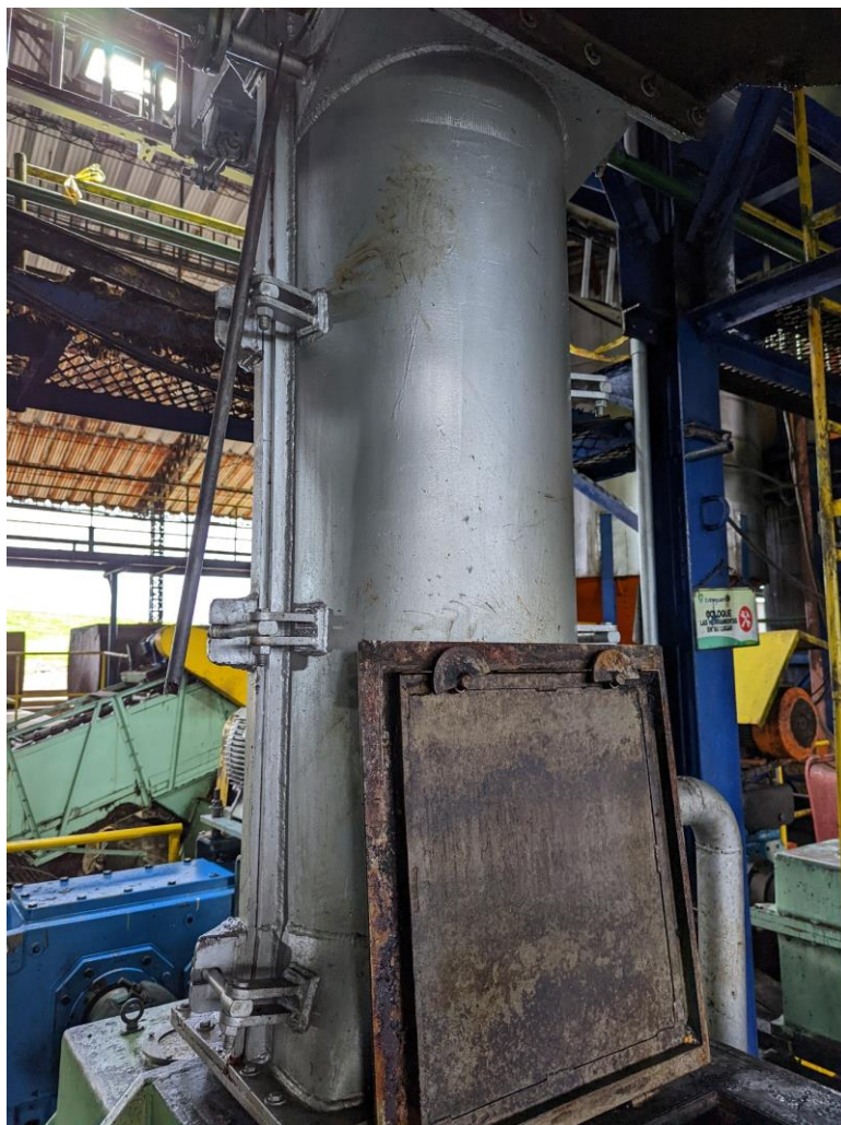
Figure 5 New conditioner unit installed to process kernel-less fruit bunches
